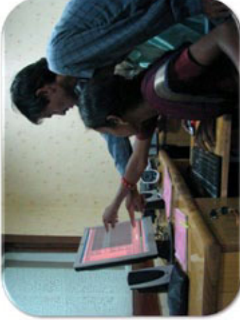
Control Room, Lalit Lokvani CR, Uttar Pradesh
